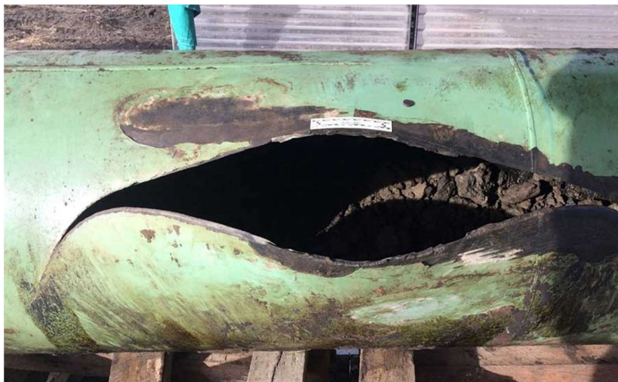
Figure 1. 4. Fatigue crack of a pipeline (source: https://www.ishn.com/articles/108930-fatigue-crack-cause-of-pipeline-rupture-oil-spill )
