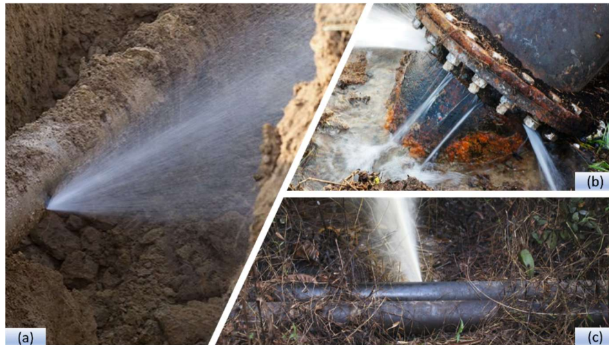
Figure 1. 2. Uncontrolled pipeline leaks (sources: (a) https://www.torque-lock.com/dont-ignore-water-damage-warnings/ , (b) https://www.siliconrepublic.com/machines/mit-pipeguard-water-leaks , (c) https://www.cfr.org/blog/trouble-oil-pipelines-nigeria )
