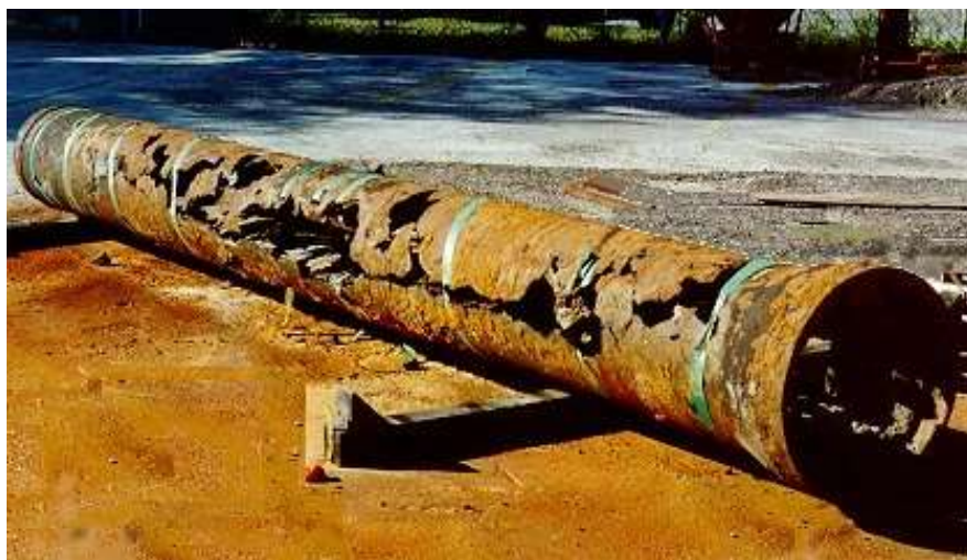
Figure 1. 3. Example of corroded pipeline (source: https://www.petroskills.com/blog/entry/00_totm/aug20-sub-oilfieldcorrosion#.YV0-qppByUk )
