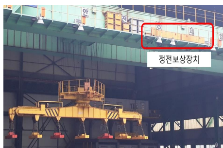
[Figure 24] 정전보상장치(power failure compensation system) (이용석, 2019)
