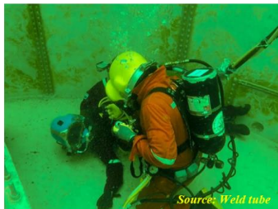
Unresponsive welder, Accident
