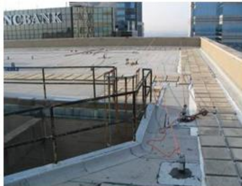
This photo shows guardrails installed along an opening. Installing guardrails early on in the construction process can eliminate the risk of a fall through an opening.
