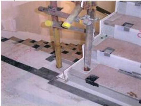
This photo shows cast sockets along the open side of a stairway. The sockets make it convenient to install temporary or permanent guardrails.
