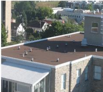
Figure 1 Planning the construction and future maintenance of a building can identify areas where permanent anchors should be installed.
