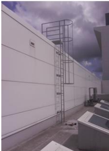
Fixed ladders should be specified to access a work platform, mezzanine, upper level, or a roof.
